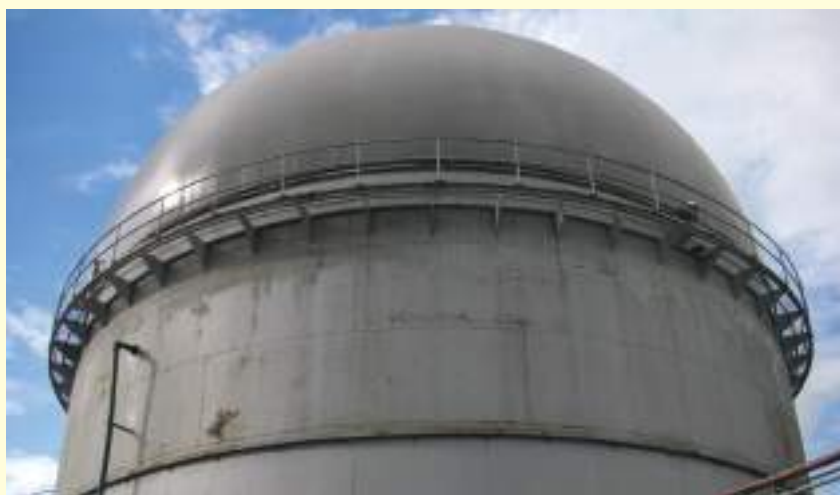
Biogas Reactor at Felda Serting Hilir
